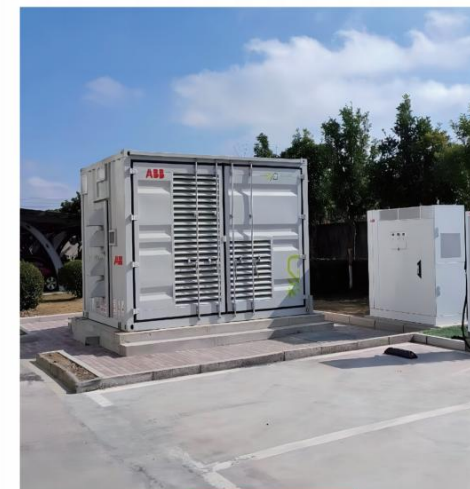
Solar Energy Storage & EV Charging Project in Lianzhuang ABB Park
