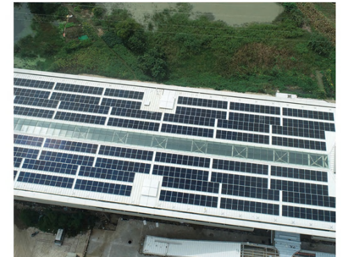
The rooftop distributed PV power plant of light rail transit station in Wuhu, Anhui Province
