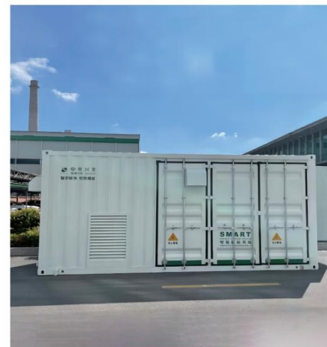
Energy Storage Project of China Power
