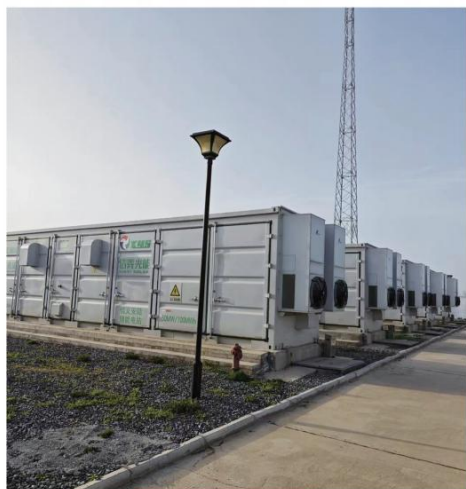
Independent(Shared) Energy Storage Power Station in Anlu,Hubei
