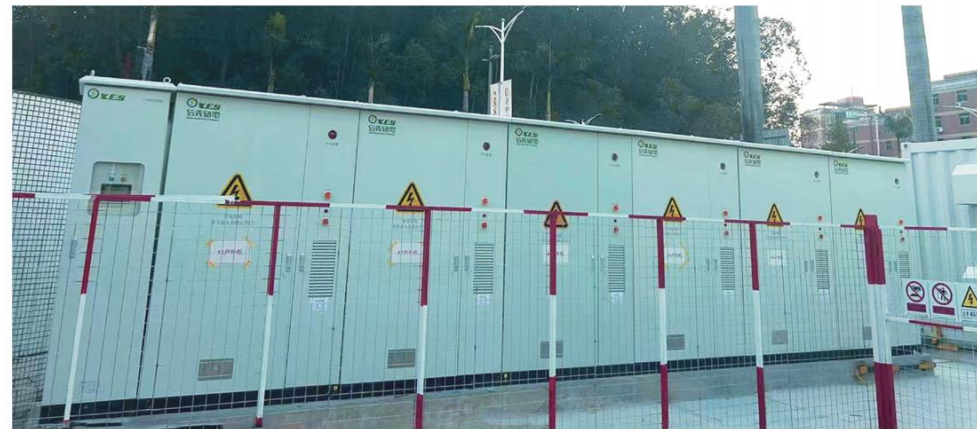
Energy Storage Project in Henggang Shenzhen
