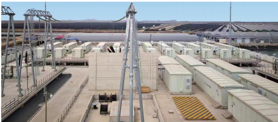
Energy Storage Power Station of CR Power in Caofeidian
