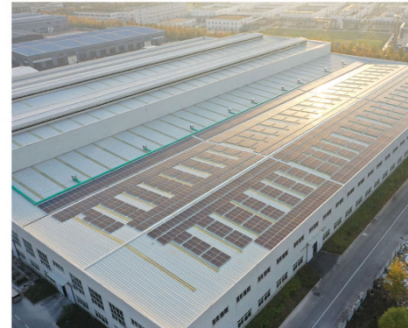
The rooftop distributed PV power plant of Jiangsu Xunai
